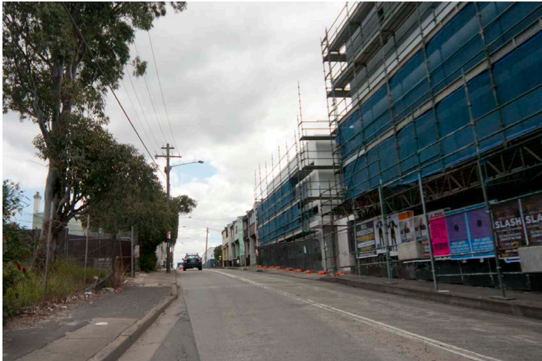
Figure 157: Campbell Street St Peters looking north towards the Princes Highway – modern residential flats under construction with circa 1880s terraces beyond (Sub Area 8)
